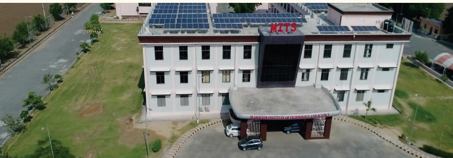
Contributing towards better environment- Solar power plant installed in the campus of MITS
